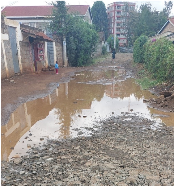
Figure 39 - Current Roads Condition
