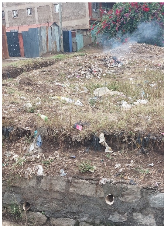
Figure 13 - Poor sewage and solid wastes disposal
