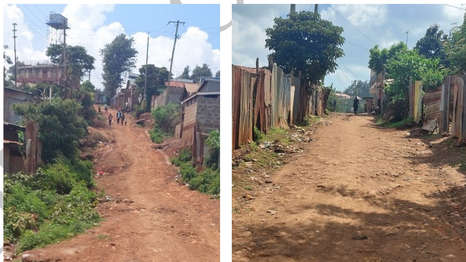
Figure 26 - Current Road Condition
